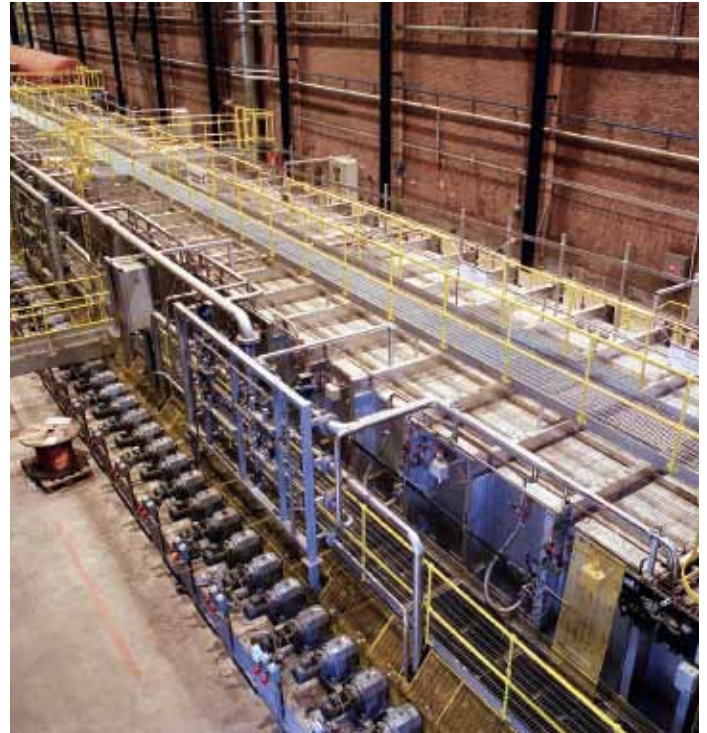
Roller hearth heating furnace with REBOX® oxyfuel solution including ceramic oxyfuel burners and Linde control system
