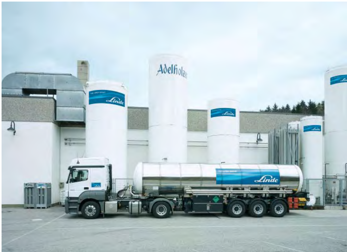
New delivery for the drinks industry. The gases are stored in special tanks before being deployed in various production processes.
