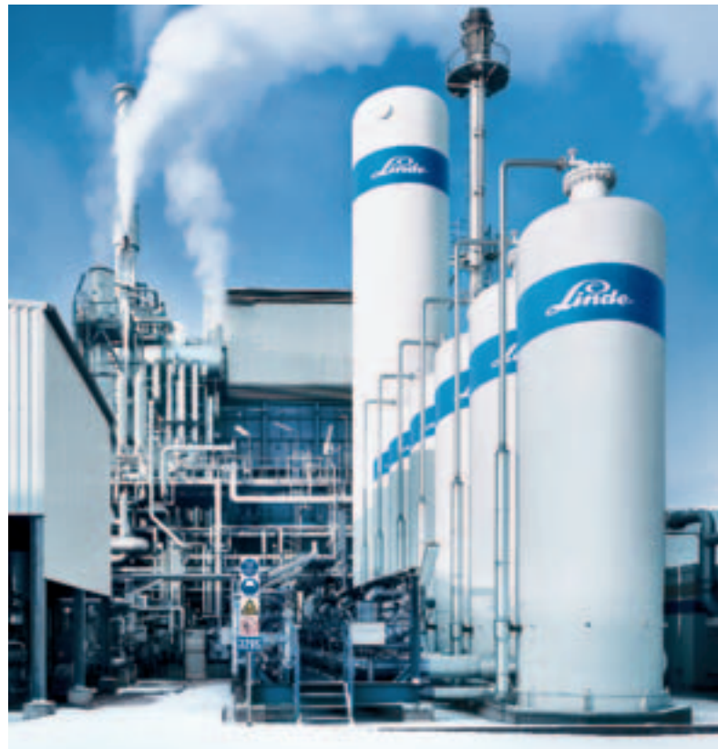
Steam reforming plants from Linde (such as this steam reformer in Brunsbüttel, Germany), which supply up to 100,000 m 3 of hydrogen per hour, are constructed for various capacities. Linde exports technology for steam reforming plants throughout the world, e.g. to the USA, the Middle East, Russia, Canada, India, Japan, China and the EU countries.
