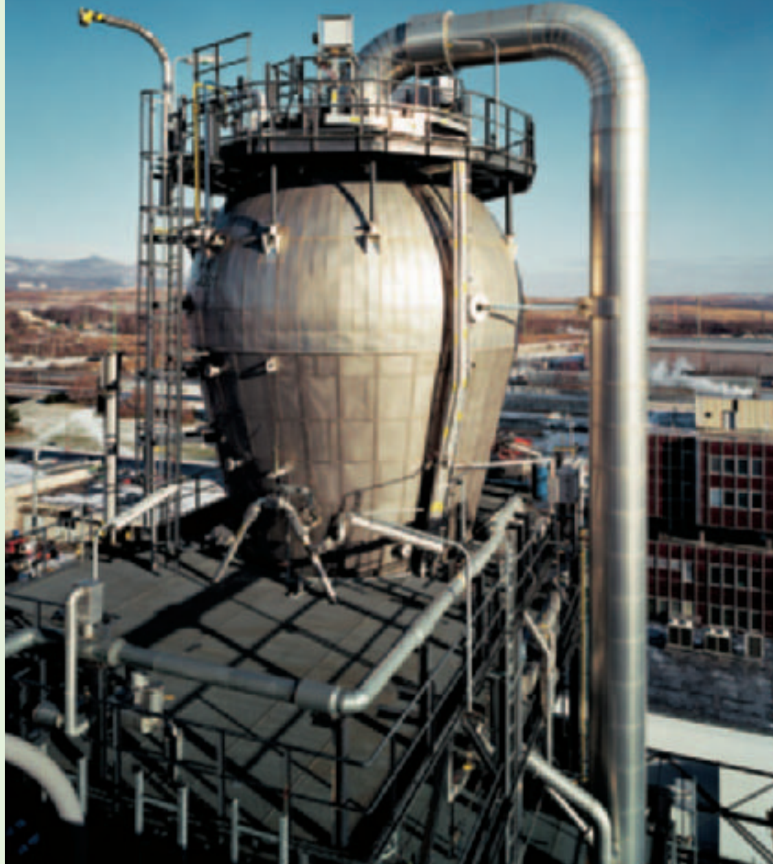
The art of the engineer is in the detail: This polymerization reactor is at the heart of a polyethylene plant built jointly by Linde and its partners in the Czech town of Litvinov which produces 200,000 tonnes of plastic every year.
